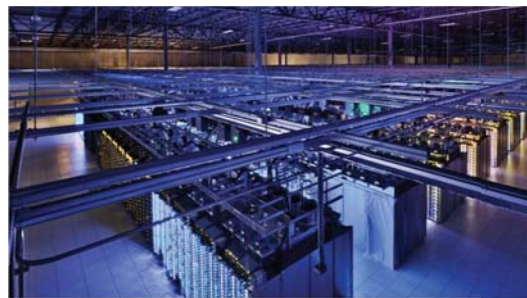
Data Center Cooling
